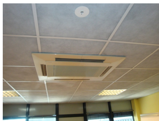
Figuur 5: Plafondunit airconditioning.
